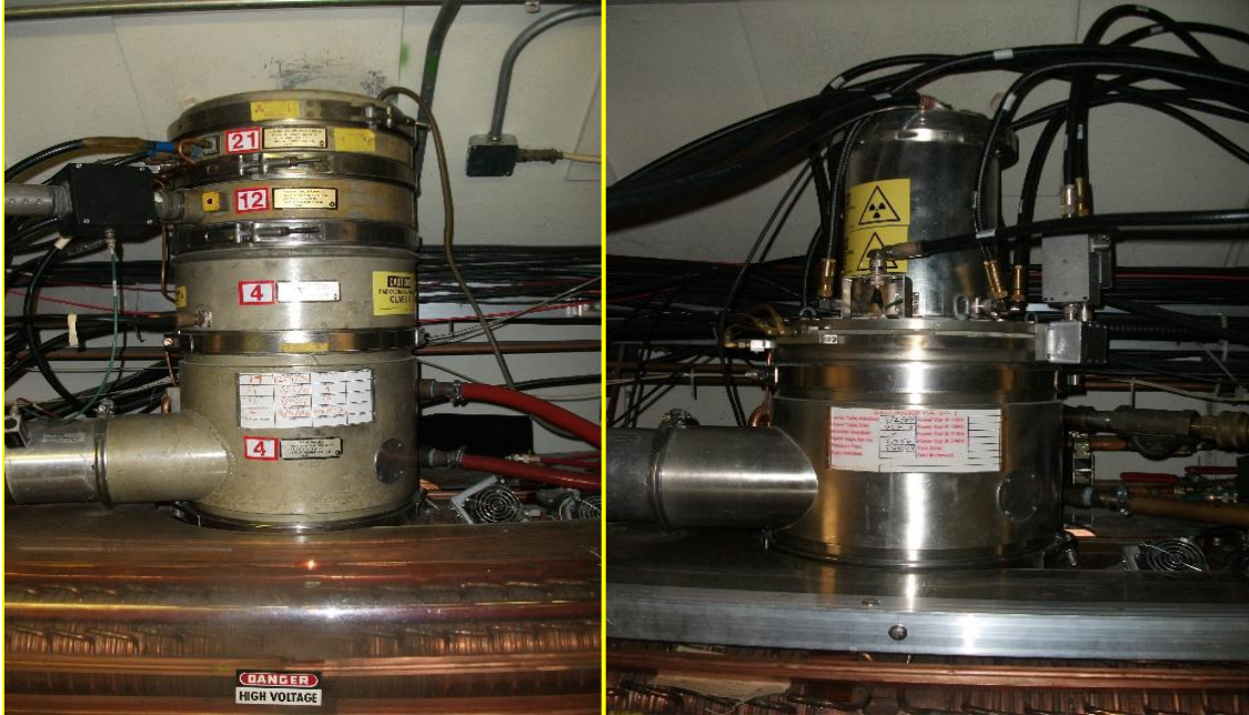
Figure 6. Forty year-old Power Tube Amplifier (left) and the replacement solid state unit (right)
